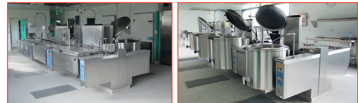
Central kitchen - Georges SAND hospital - Bourges (18)
